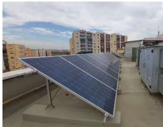
Solar panels installed on the roof
