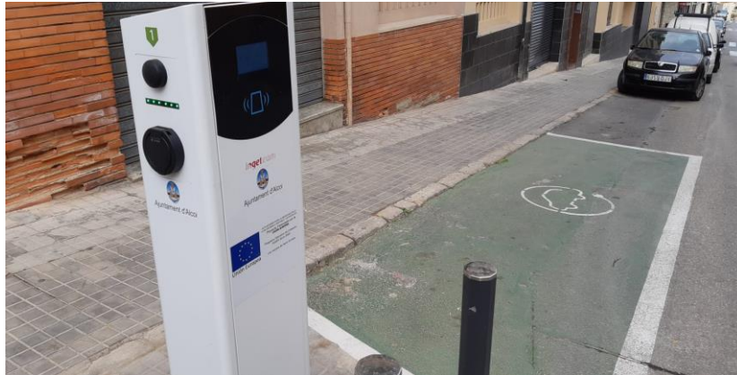
One of the electric chargers on a side street off Entenza
