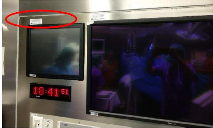
Integrated Operating Room Panel at Pediatric surgical block
