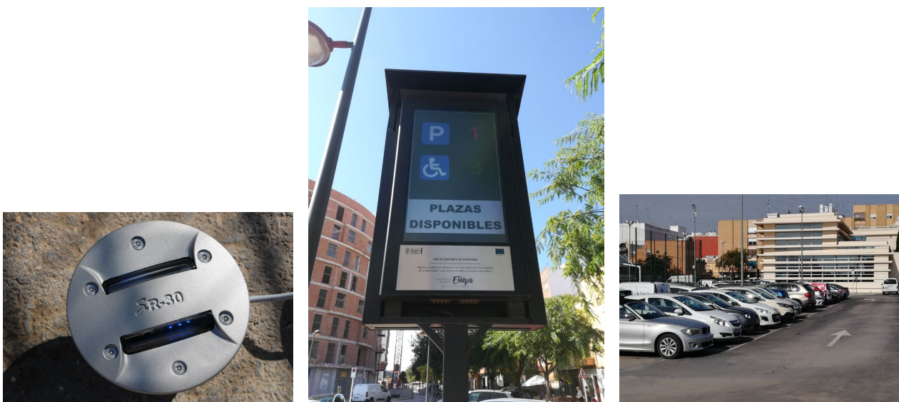
SENSOR, ELECTRONIC PANEL AND PARKING AREA
