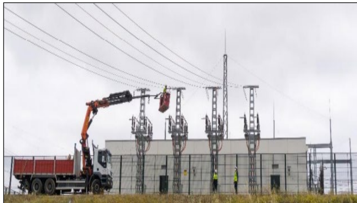
Electrical substation of Cañaverall (Cáceres)
