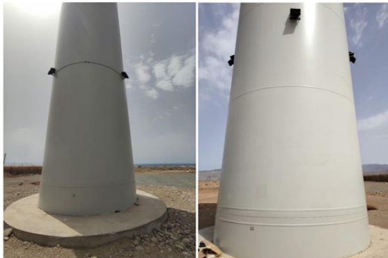
La Caleta Wind Farm - Probird System Photo Courtesy of ECOENER
