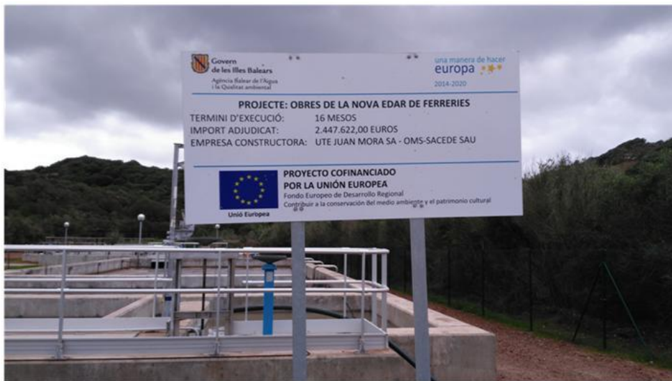
Informative poster of the construction works of the new Ferreries treatment plant
