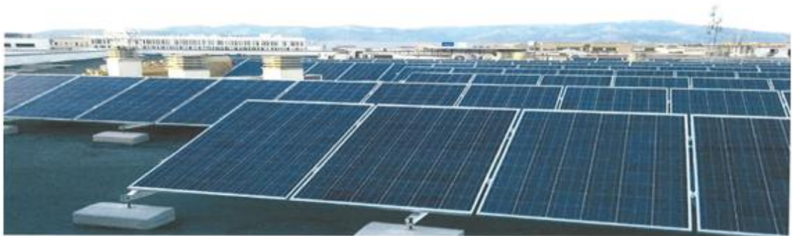
Image of the solar panels installed in the company Salabert e Hijos, S.A.
