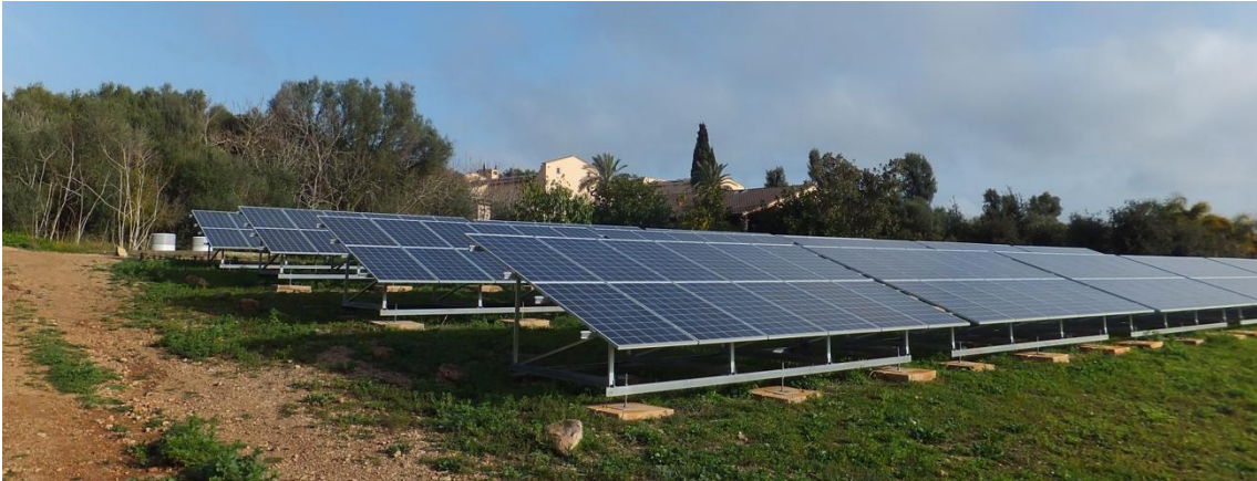
Image of the solar panels installed in the company Finca Es Fangar, S.A
