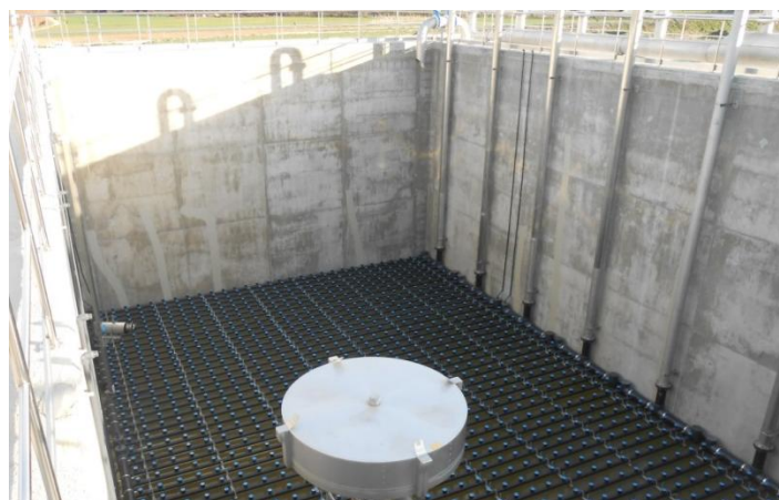
Interior reactor CLEARGREEN
